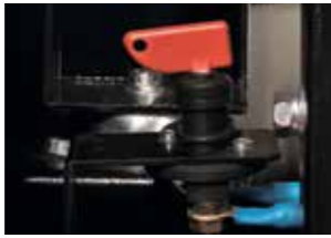
Main battery switch
