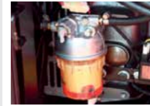
Diesel filter with water separator
